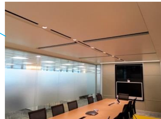
Chilled Ceiling Panel at Meeting Room
