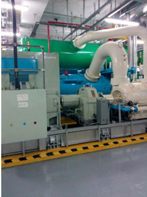
Chiller Before Replacement
