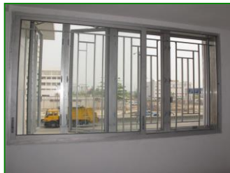
Acoustic Window (-6.4dBA)
