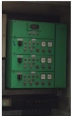
Electrical Distribution Equipment
