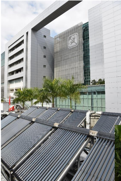
Solar hot water panel
