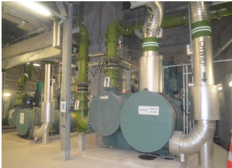
The installed 1.4MWr and 4.3MWr Chillers at the North Plant
