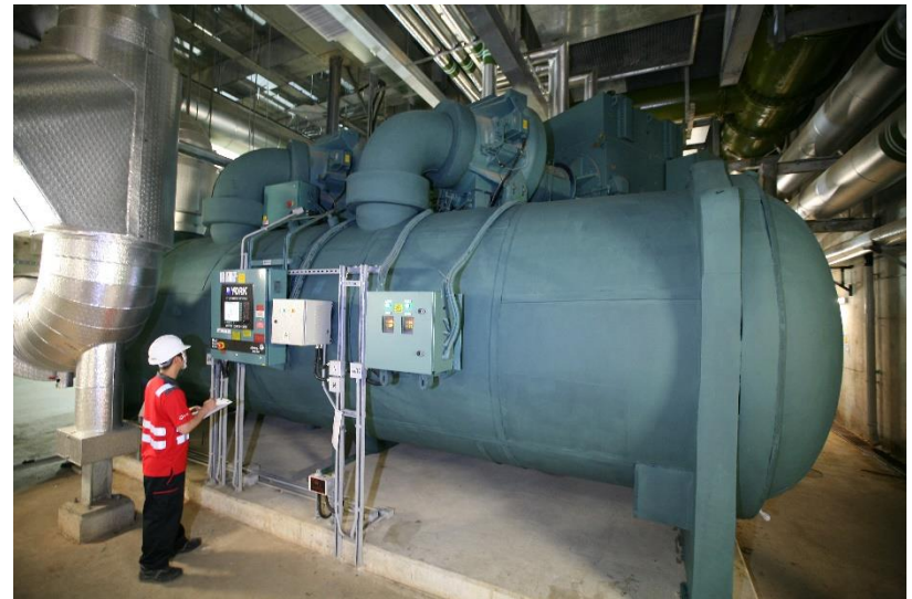
The installed 17.5MWr Chiller at the South Plant
