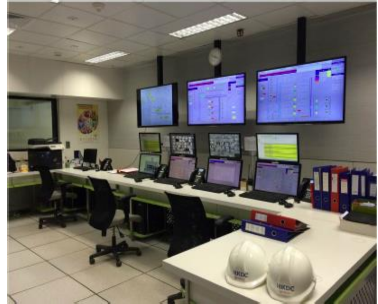
DCS Control Room
