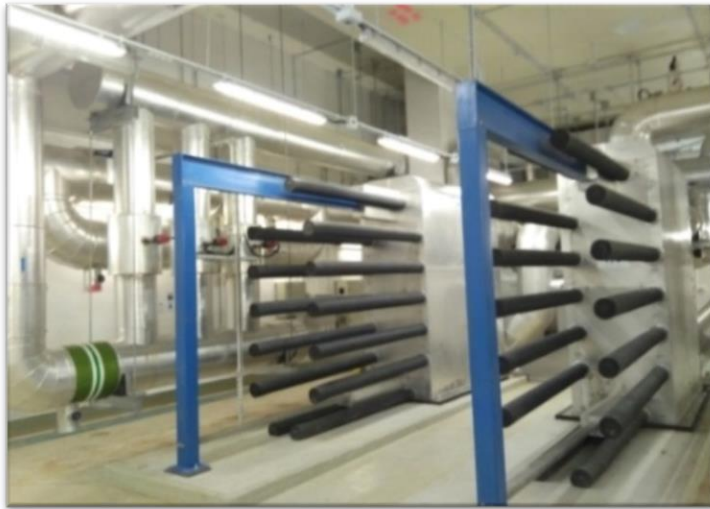
Heat Exchangers in DCS Substation
