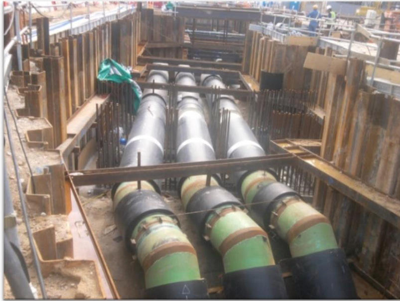
3-Pipe System of Underground Chilled Water Piping in Open Trench
