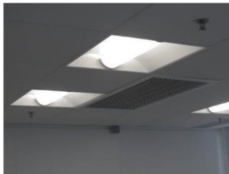
High efficiency lighting at office area
