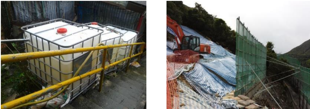
Figure 5: Water pollution control measures (left photo) and air pollution control measures (right photo) for the LPMit works
